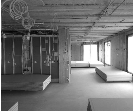
Figure 4: Picture during construction of an apartment prior to the dry-walls. SOURCE: Antinnen Oiva Architects
