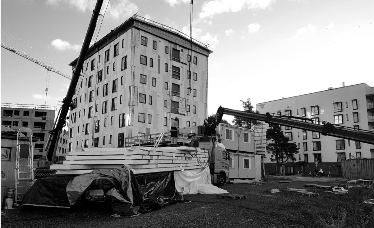
Figure 2: Construction crew at work unloading a truck at Lighthouse Joensuu site. Courtesy of Rakennustoimisto Reijonen
