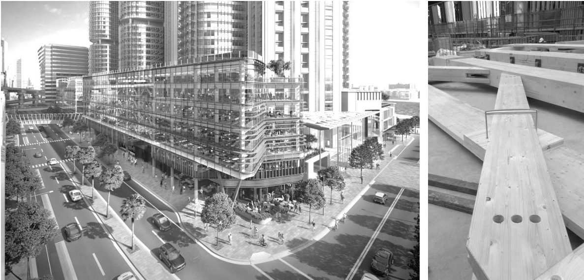
Figure 3 and 4: Daramu House (“tree house” in local Sydney aboriginal language), under construction at Barangaroo
