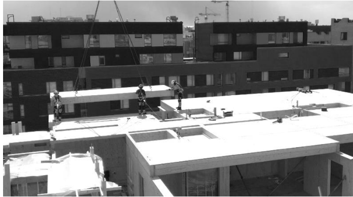
Figure 5: Picture during assembly of the structural elements: LVL massive compartment walls and LVL Rib Panels for floors.
