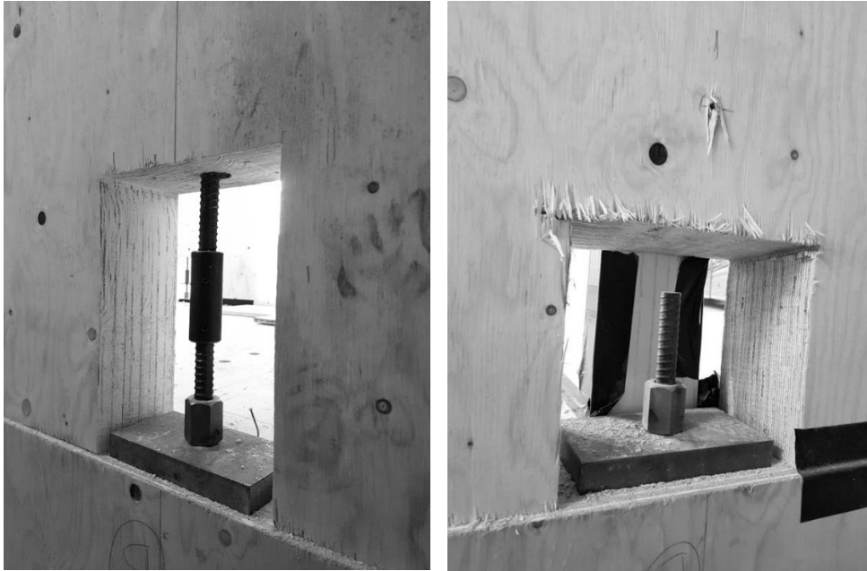
Figure 6: Restraining done from top of the wall with LVL-X wall installed afterwards. Courtesy of Rakennu-stoimisto Reijonen
