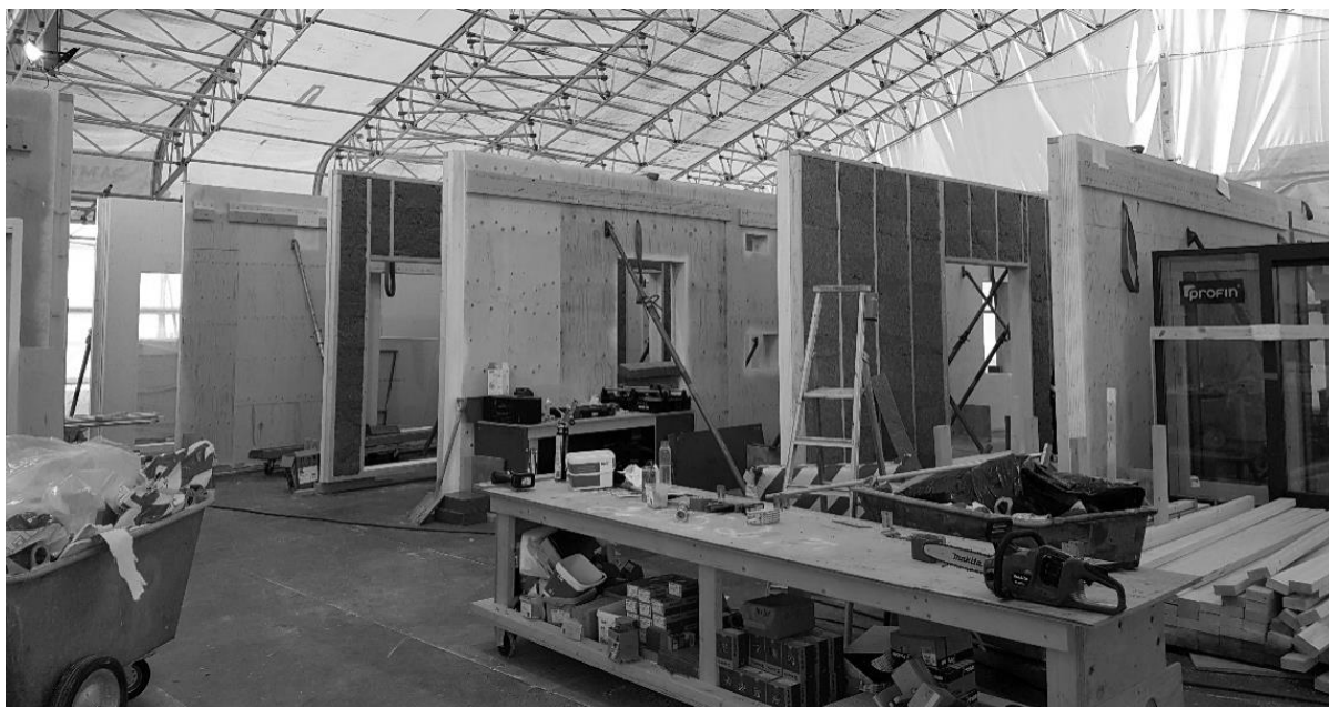
Figure 9: Picture taken from inside of the prefabrication tent located next to building site. Courtesy of Rakennustoimisto Reijonen
