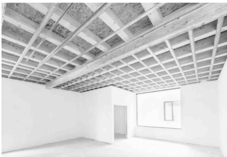
Figure 9: internal view of the spaces with plasterboard walls and the counter ceiling ready to be put in place
