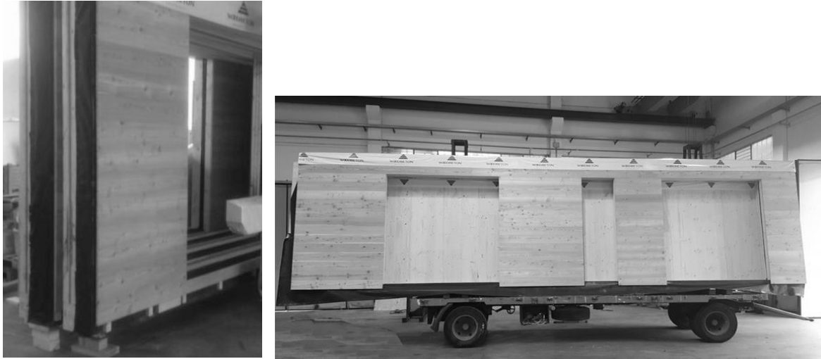
Figure 4+5: Prefabrication of the wall in the factory with cladding and transport to the building site.
