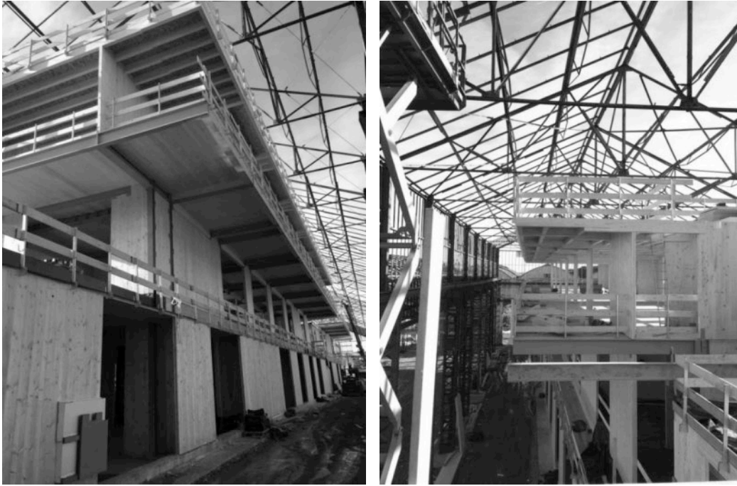
Figure 6: some pictures of the building on site during the installation of the timber structures
