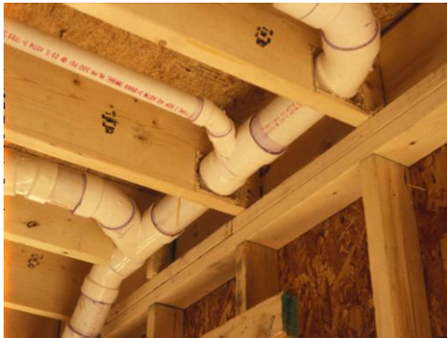
Figure 5: Improperly cut, notched and drilled floor joists by plumber.
