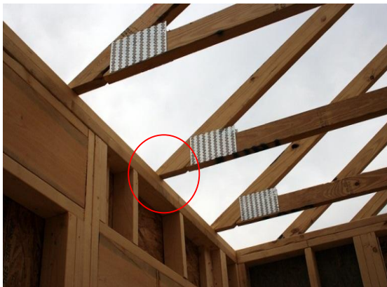
Figure 6: Improper truss support.
