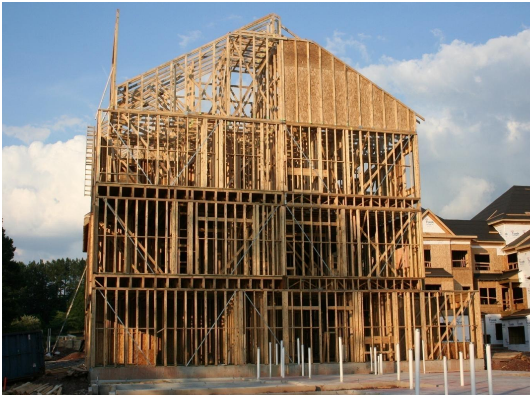
Figure 3: Platform frame building showing the second and third floors built on top of the wall studs. Sheathing of plywood or OSB is will be installed on the floors, outside walls and roof.
