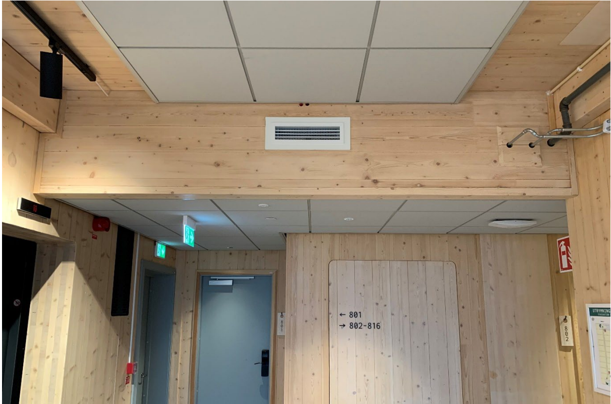
Figure 12: Typical implementation of technical systems. Photo by Mark Wojcik
